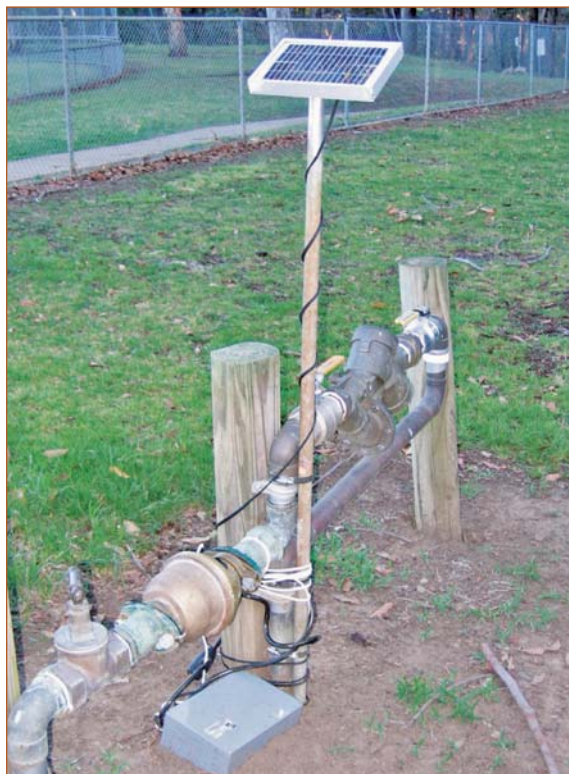
Figure 6. Example of a field installation of a standalone smart water meter.
